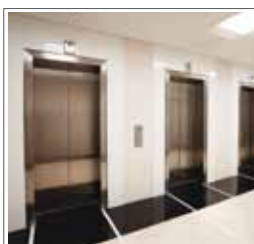
Ascensoristica Elevator sector
